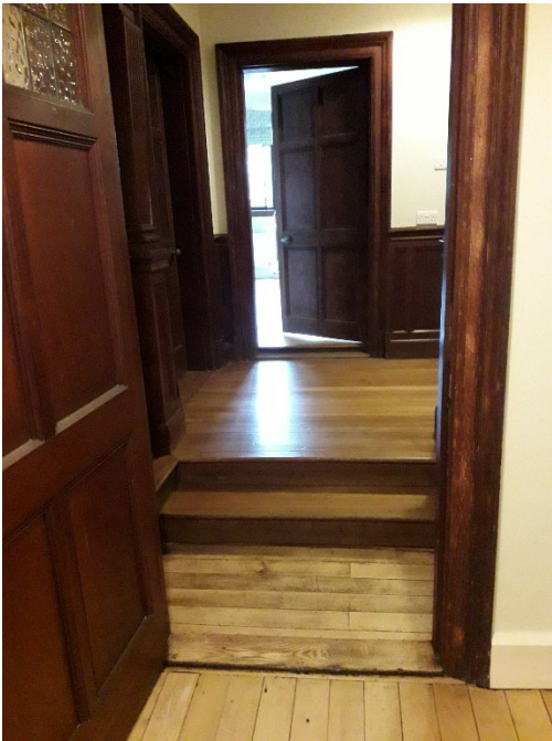
Apartment internal main entrance door, looking in from external lobby – showing two steps down & threshold inside.
