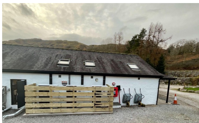
Air source heat pump enclosure at Eskdale Campsite.
