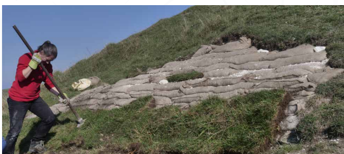
▲ Erosion can be a significant problem on historical earthworks. It requires prompt recording and action before it gets out of hand.
