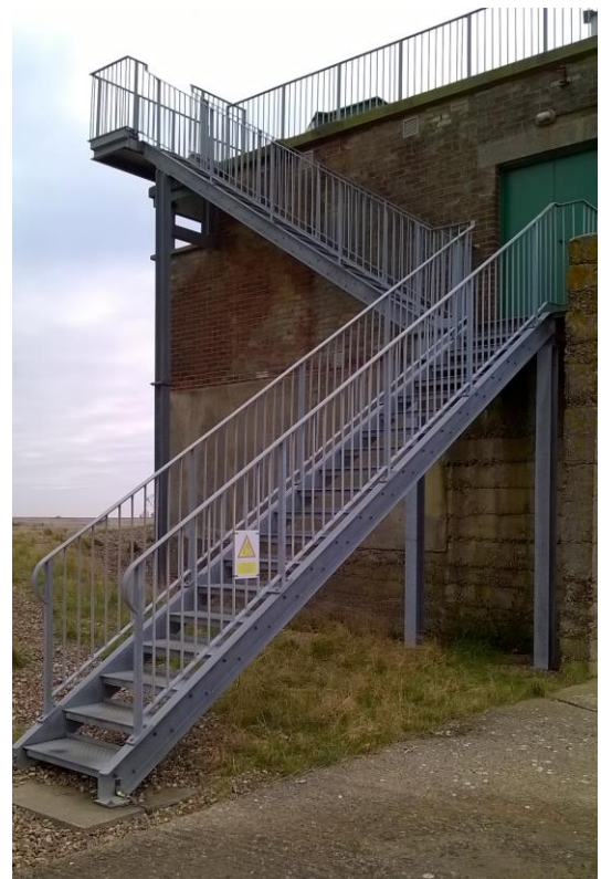
Steps to the main floor and roof of the Bomb Ballistics building
