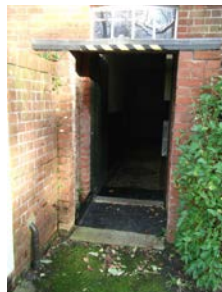
Side entrance door
