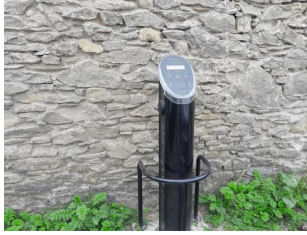
Electric charging point
